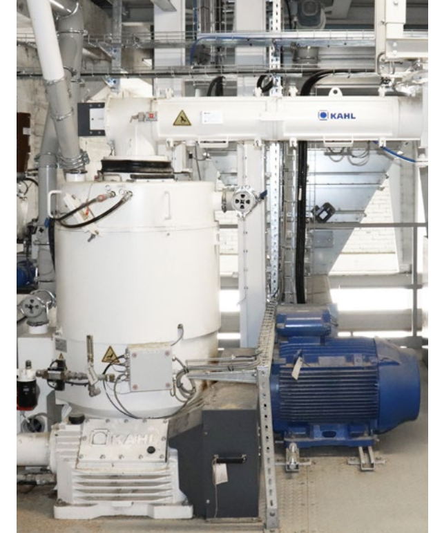
The flat die pelleting press is already in operation at the Ziegenaus Bennomühle mill in Friedberg, Southern Germany.
