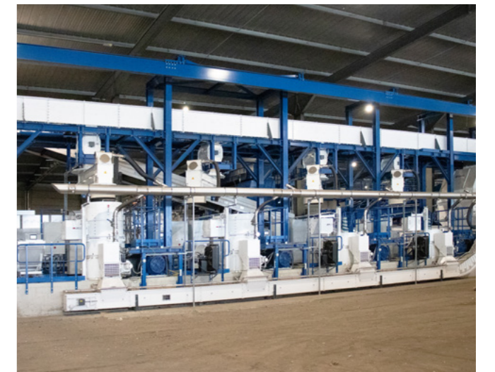
↑ Recycling plant with a throughput of 85 000 t/a
